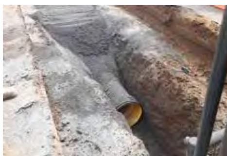
PICTURED: Top; new concrete footpath at Bailey Park. Above; a new wastewater treatment system will service Bailey Park; watermain replacement was completed trenchless technology.
