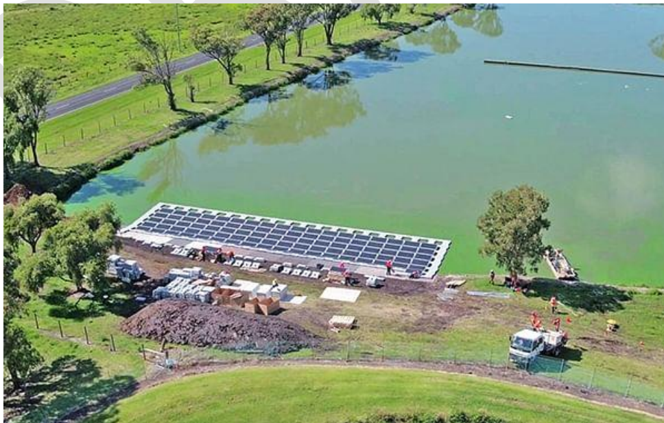
LISMORE CITY COUNCIL'S FLOATING SOLAR ARRAY THROUGH 'FARMING THE SUN'
